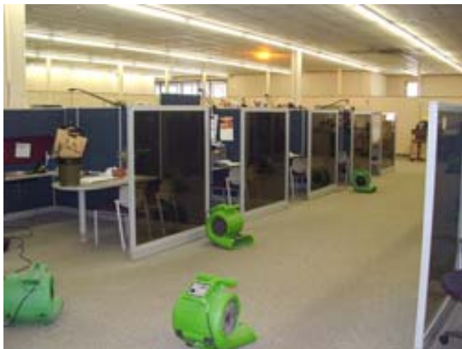
Blowers were set out to help dry carpet in the flooded Charleston WORKFORCE West Virginia Center.
