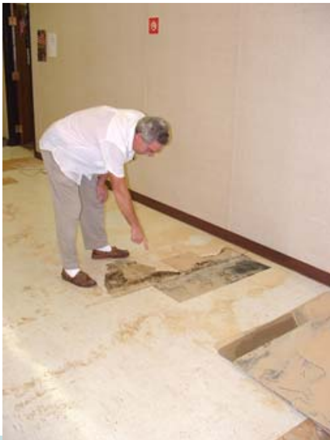
FAM/MIS Warren Wingo points to damage in and under the floor after water flooded up from beneath.
